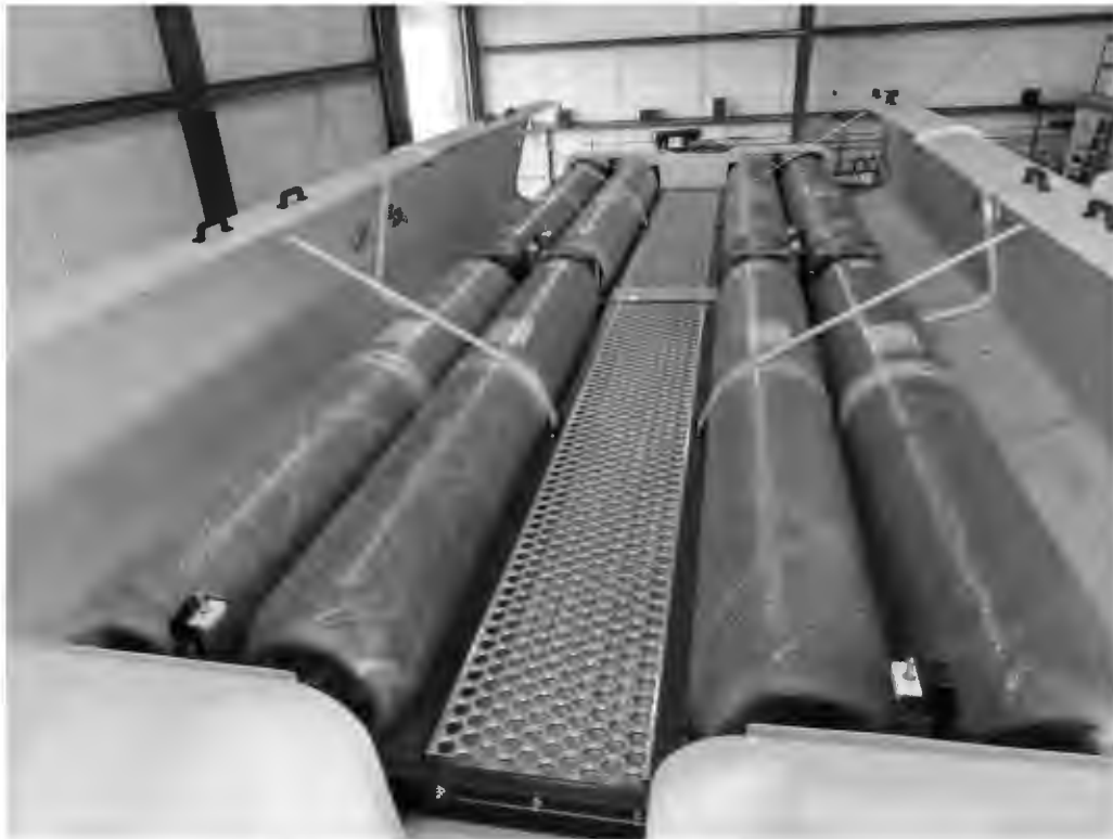
ROOFTOP CNG TANKS
