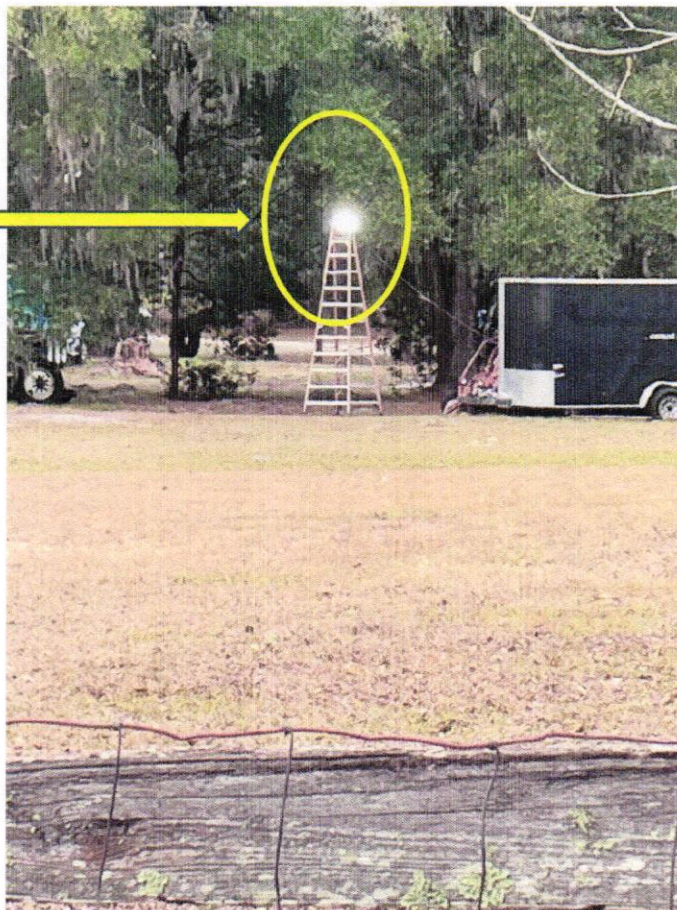
Industrial light mounted on tall ladder... By Day
