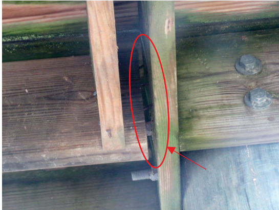
Exhibit 9 – Separation of end-nailed joist connection
