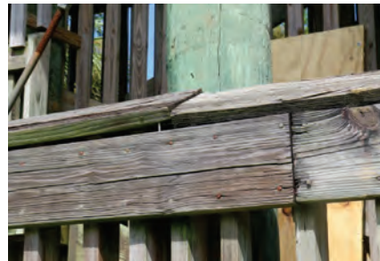
Exhibit 3 – deteriorated railing components
