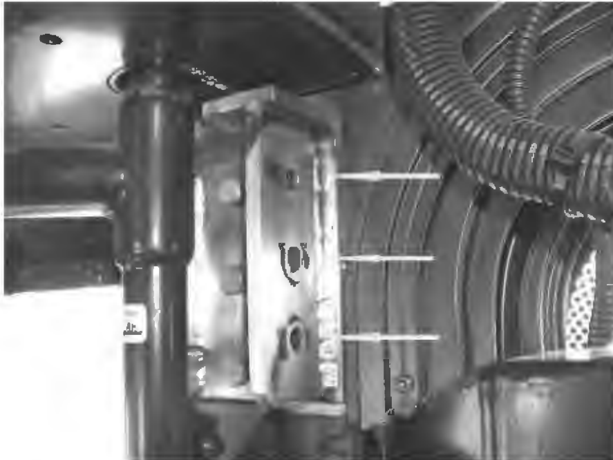
BROKEN BOLTS FRONT DOOR; UPPER SUPPORT BRACKET (13,877 TEST MILES)
