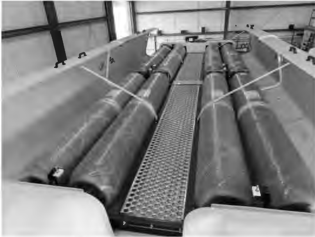
ROOFTOP CNG TANKS
