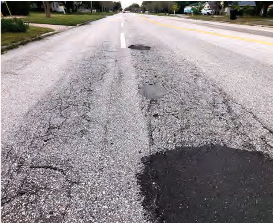
62nd Avenue NE Pavement Conditions
