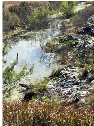
Waste in Drainage Ditch
