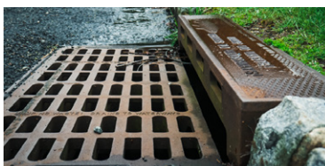
Storm Water Drain
