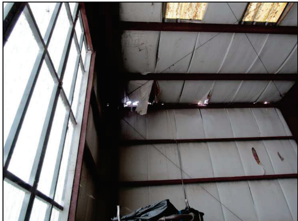
VIEW OF CEILING INSULATION & POSSIBLE LEAK AREA
