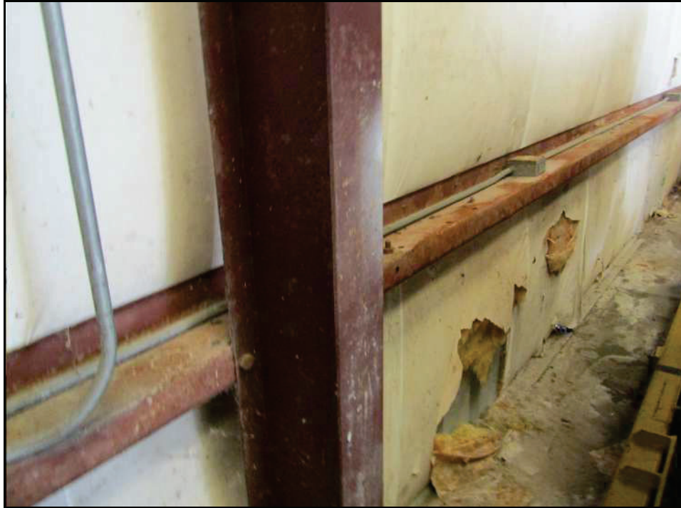
VIEW OF WALL INSULATION & PITTED STEEL BEAMS
