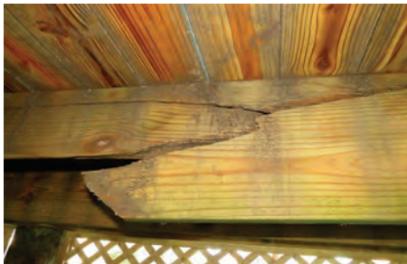
Exhibit 2 – section loss/separation along deck joist
